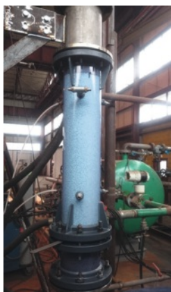
Fig. 6. Industrial pilot plant for pressure drop measurement.
