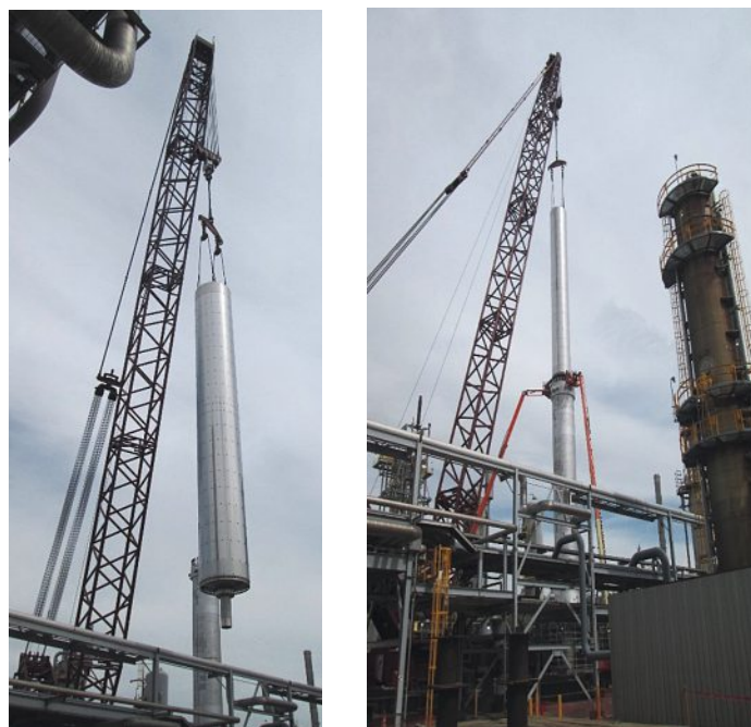
Fig. 9. Cartridge lift and installation inside converter.
