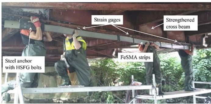
Fig. 11. Installation of Fe-SMA on a steel bridge as prestressing members. Reprinted from Engineering Structures 2021, 248, 113231. Copyright (2021), with permission from Elsevier.
