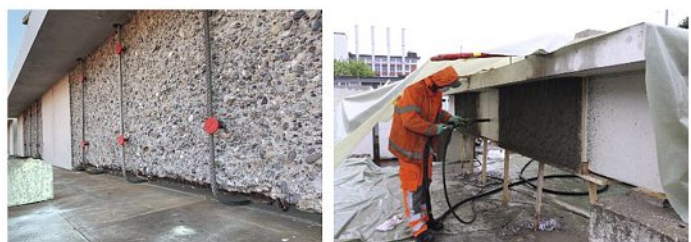
Fig. 6. Shear strengthening of RC beams using Fe-SMA: (a) u-shaped stirrups; (b) embedment in a mortar layer. Reprinted from Construction and Building Materials 2021, 274, 121793. Copyright (2021), with permission from Elsevier.
