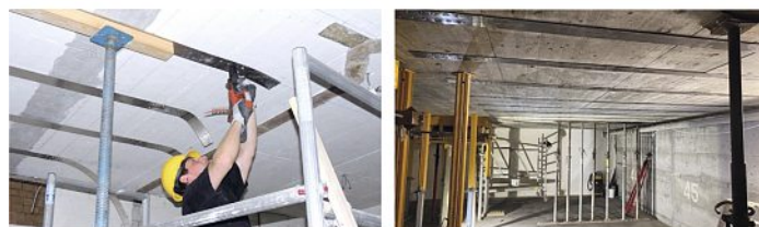
Fig. 9. Pilot application with re-plate in 2017 (left) and strengthening in a parking garage in Nussbaumen in 2020 (right)
