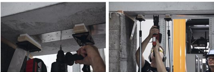
Fig. 5. Flexural strengthening of RC slabs using externally unbonded Fe-SMA strips. Reprinted from Structural Concrete 2018, 19, 876. Copyright (2018), with permission from John Wiley and Sons.
