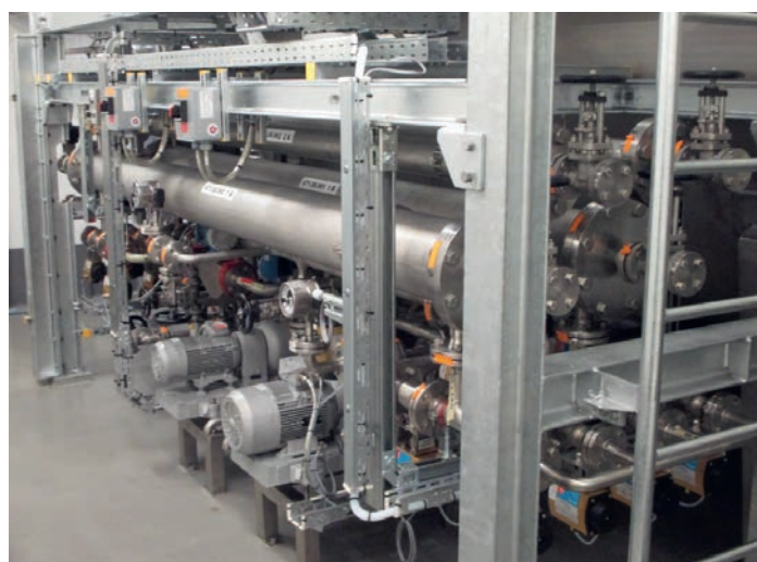
Fig. 4. Nanofiltration unit for selected biotechnology WWs at Roche Basle. Photo©Roche Basle.
