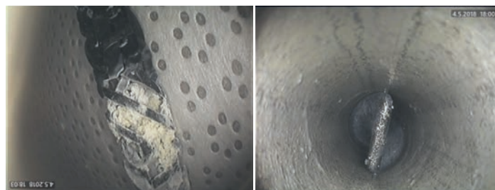
Fig. 12. Visual inspection after run 1. (left) X-type static mixer removed from tubular reactor; (right) Inner view of the tubular reactor with helical static mixer located after the mixer.
