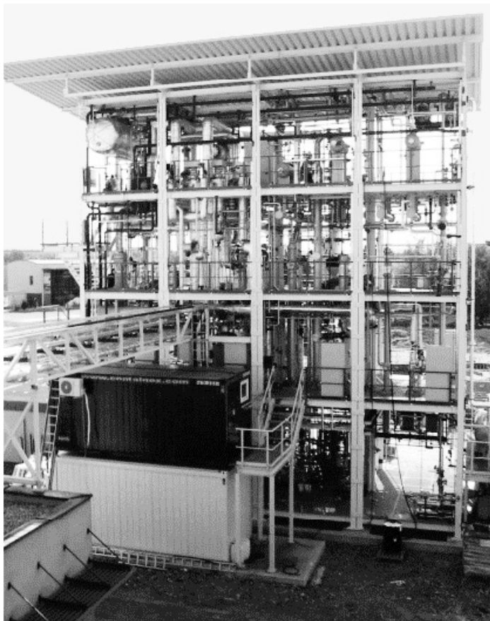
Fig. 4. The 1 MW SNG process development unit (PDU) in Güssing, Austria, converting wood-derived producer gas to SNG.
