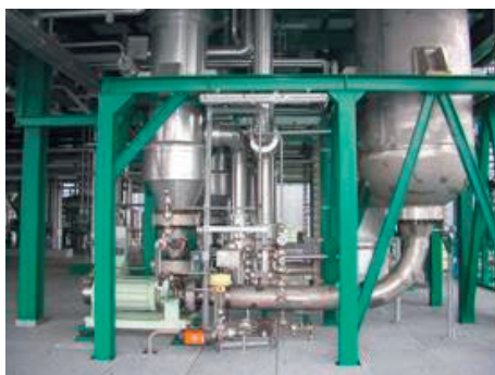
Fig. 24. Lower part of the 10 m 3 production loop reactor.
