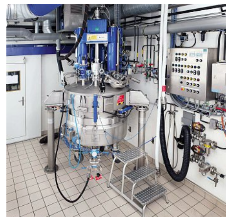
Fig. 1. 1000 L stainless steel reactor for SPPS.
