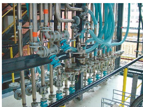
Fig. 5. Coupling station in the E13 multi purpose plant
