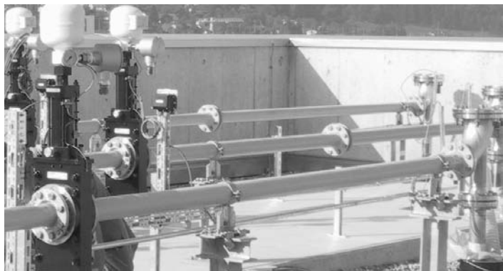
Fig. 6. Roof setup with fast-acting valves and flame interrupters
