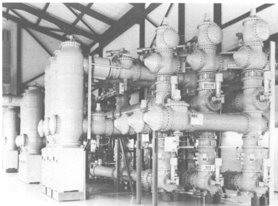
Fig. 1. High-voltage switchgear stations up to 800 kV in GIS-technology (SF 6 gas-insulated and fully enclosed) require much less space than their air-insulated counterparts
